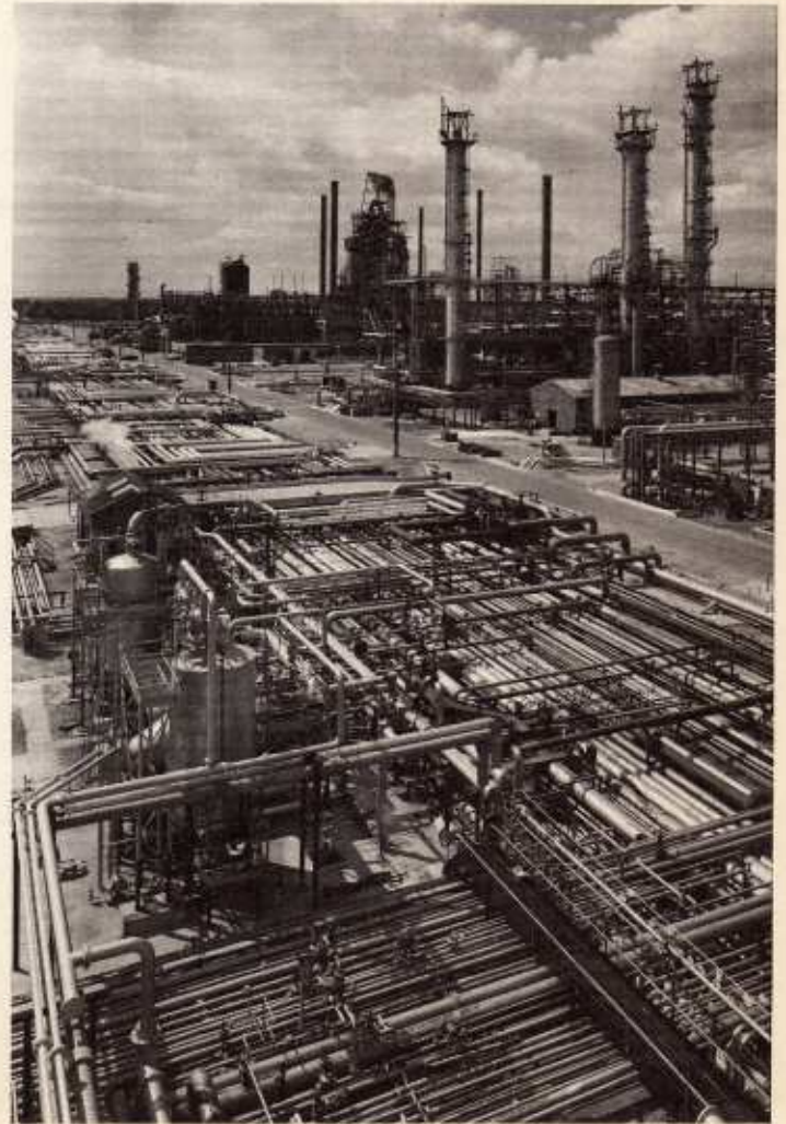
Miles of intricate piping – Stanlow Refinery in Cheshire.
