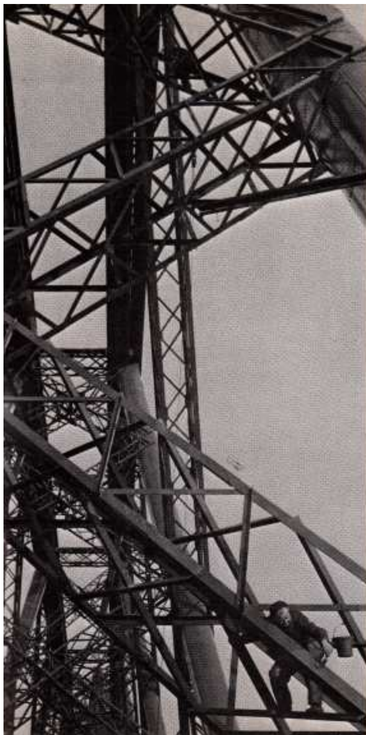
Painting is one of the commonest methods of protecting metals against corrosion. Here is a man painting the metal girders of the Forth Railway Bridge. British Railways
