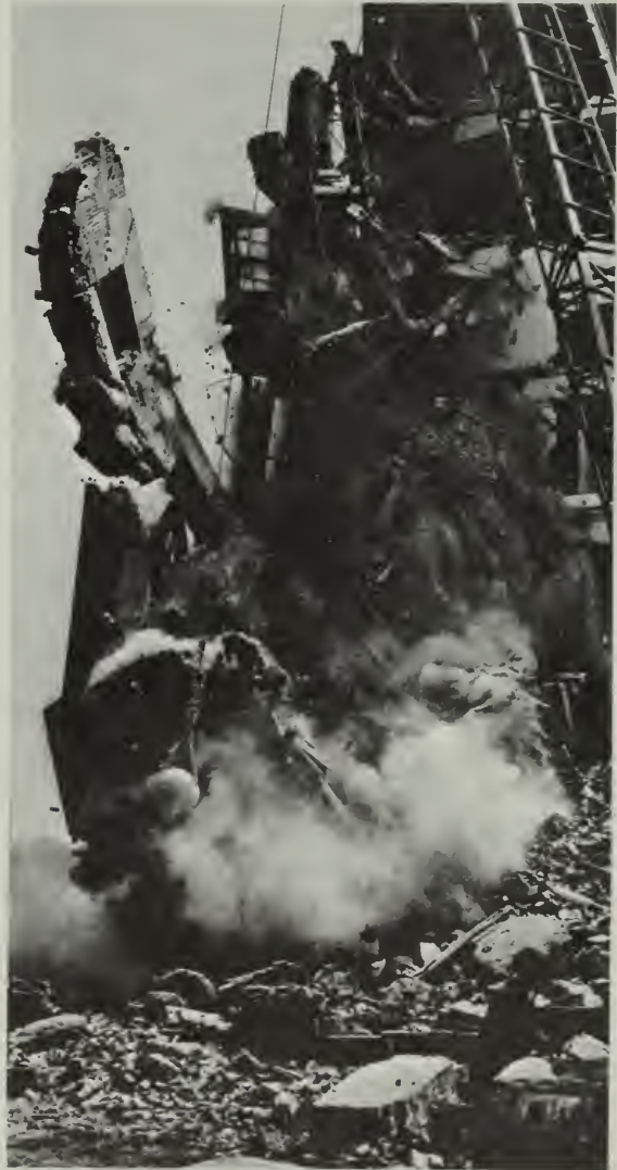
A 3,000-pound steel ball swung by a crane against the walls of a condemned building. What happens to the momentum of the ball?
