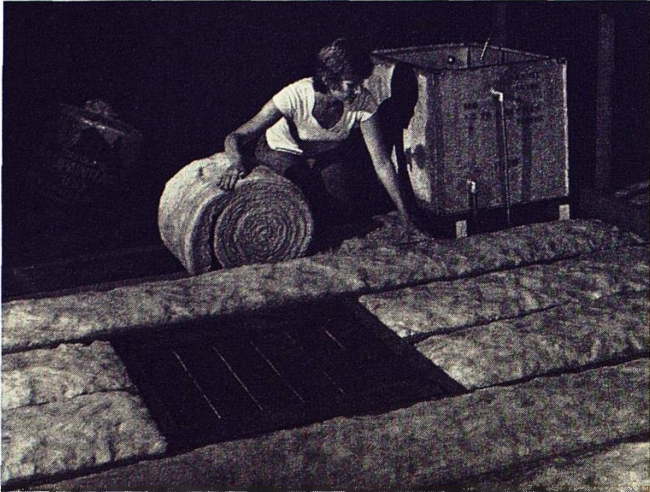
Different materials can be used to stop heat loss through roofs. Here glass fibre is being laid.
