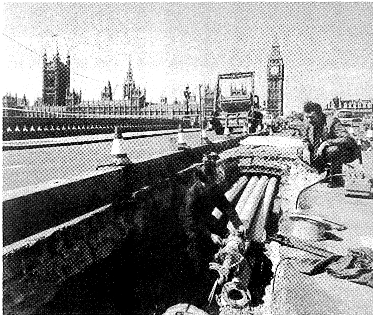
Figure 5 Local service pipes — under the roadway on Westminster Bridge
